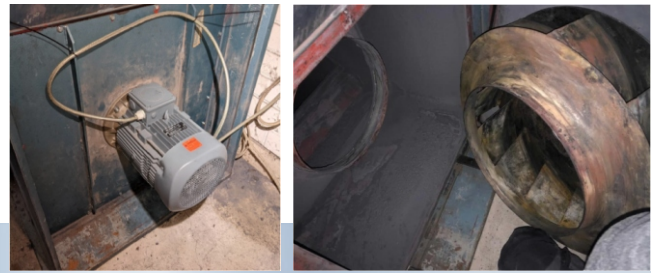
Pic. 2/3) On the left, the drive motor for the fan wheel when installed. On the right the fan wheel mounted on the drive shaft of the motor.
